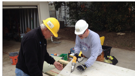
Local volunteers and City employees teamed up with Trinity Habitat for Humanity to make some much needed exterior repairs on three houses for needy families in east Arlington. Repairs included replacing trim and siding, caulking, and painting. The project was made possible with funds contributed by the Arlington Tomorrow Foundation.
